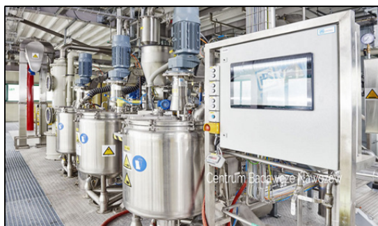
Fig. 1 Installation 1/2 technical scale for the production of microbiologically enriched fertilizers.
